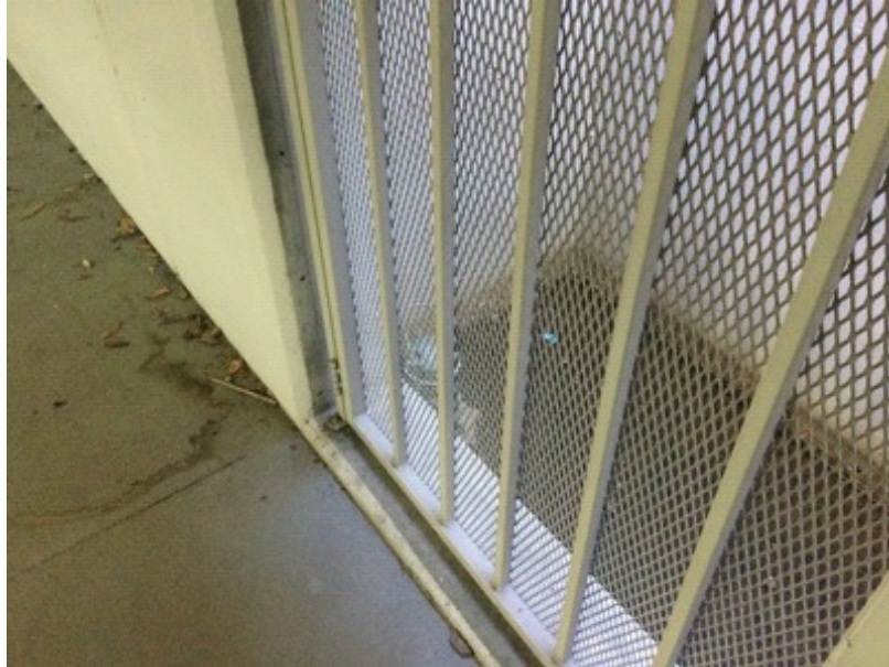
Garage sump pumps replacement has been included in the Study. The estimated useful life when new is approximately 15 years.
