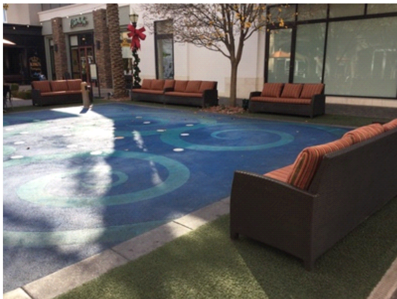
Replacement of the splash pad has been included in the Study. The cost and remaining useful life are an estimation only.
