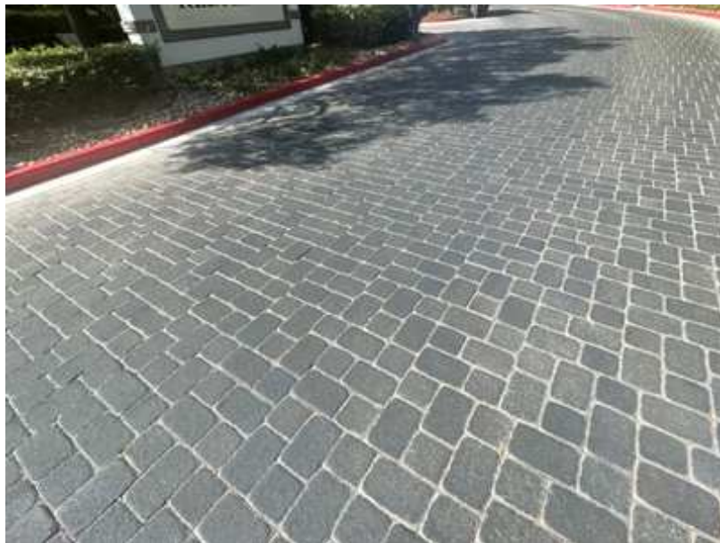
Complete replacement of all Pavers has not been included in the Study. Instead, repair and replacement has been scheduled as an allowance to be done as needed.
