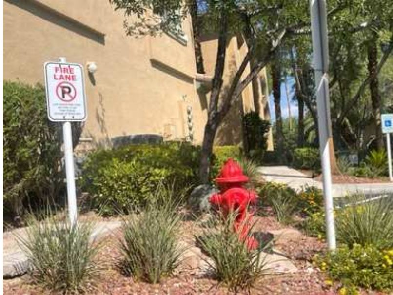
Fire Hydrants are maintained by the Association. Replacement has been included in the Reserve Study.
